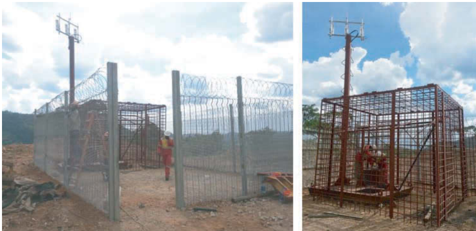
Figure 14-12 Physical Security Protecting Wireless Mesh Equipment at a Mine Site
