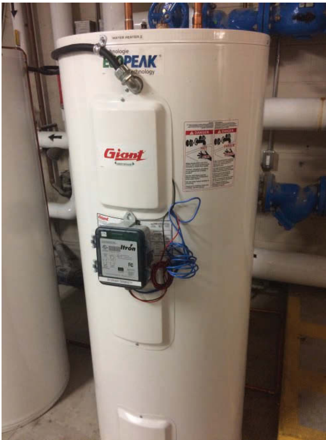
Figure 11-17 An Electric Water Heater Connected to a FAN Demand Response Controller
